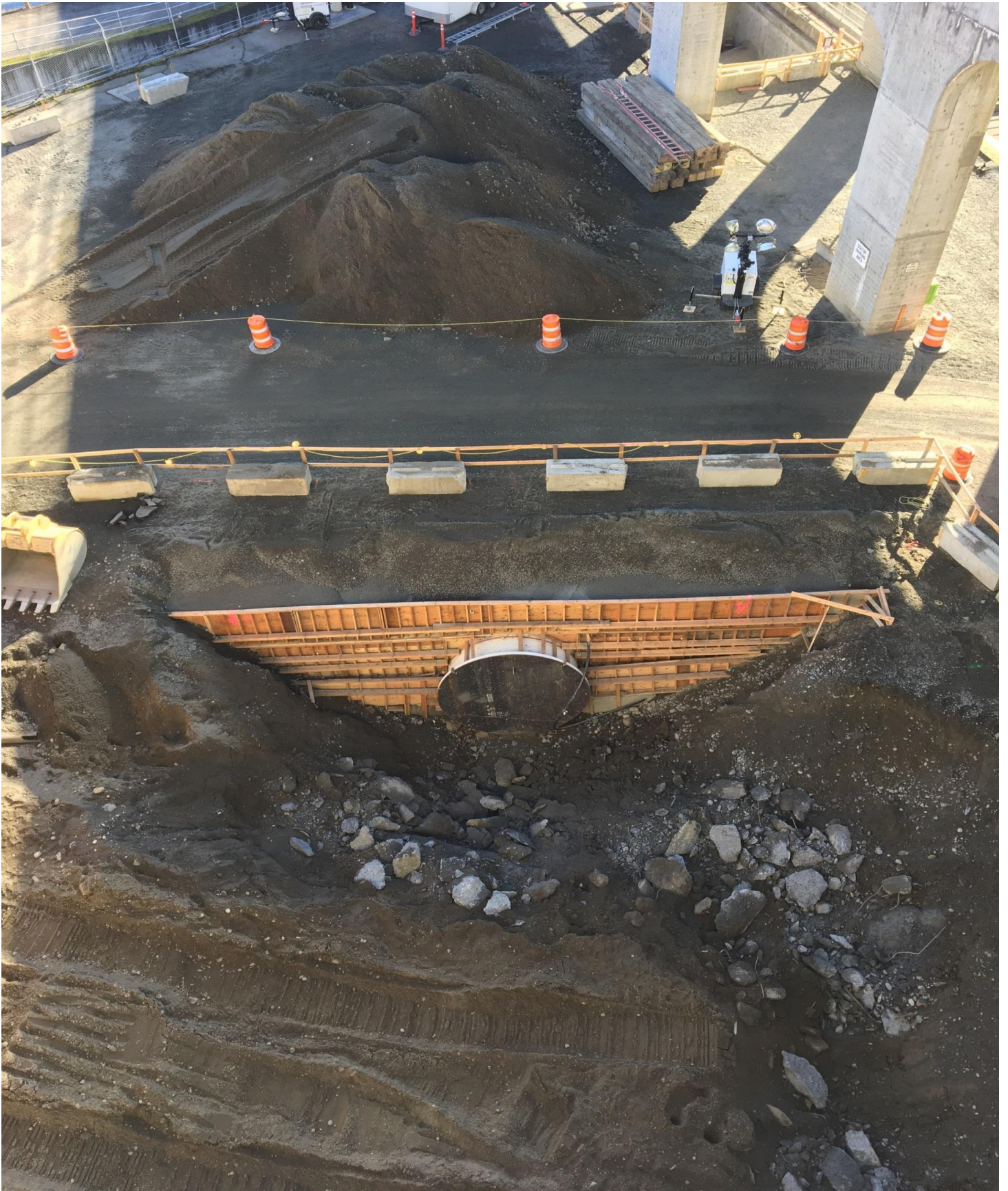
New 10' pipe section capped. Digging underway for 10" valve room at base of dam.
